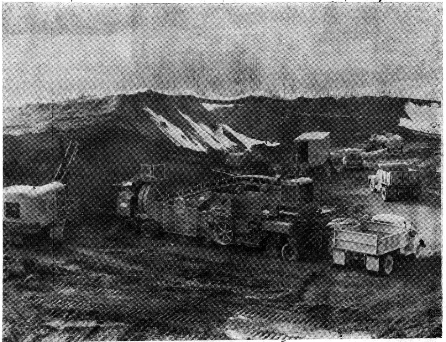
COUNTY CRUSHER — The Iron County Road Commission's new gravel crusher has been placed in operation at the county-owned pit near Stager Lake on old county road 424. A large area of the top soil has been cleared away, and the gravel underneath is being crushed and screened for use by the road crews in their 1961 road program. The area has the look of an open pit mine in miniature, with a gas shovel loading the crusher hopper, and several trucks shuttling back and forth, stockpiling the crushed gravel. (Drill photo)
